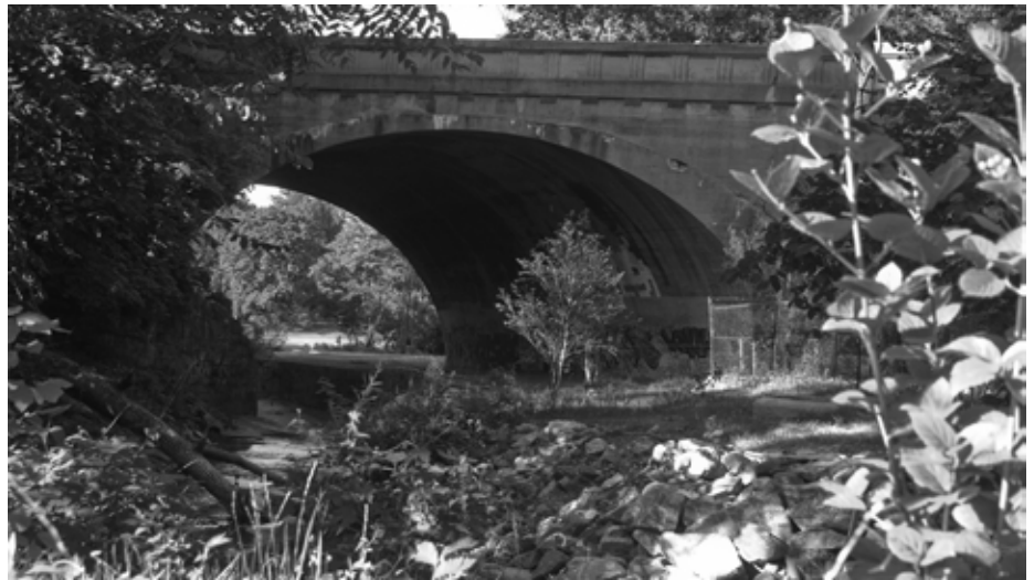
The University Parkway bridge over Stony Run will be a major passageway for the newly developed walking trail.
