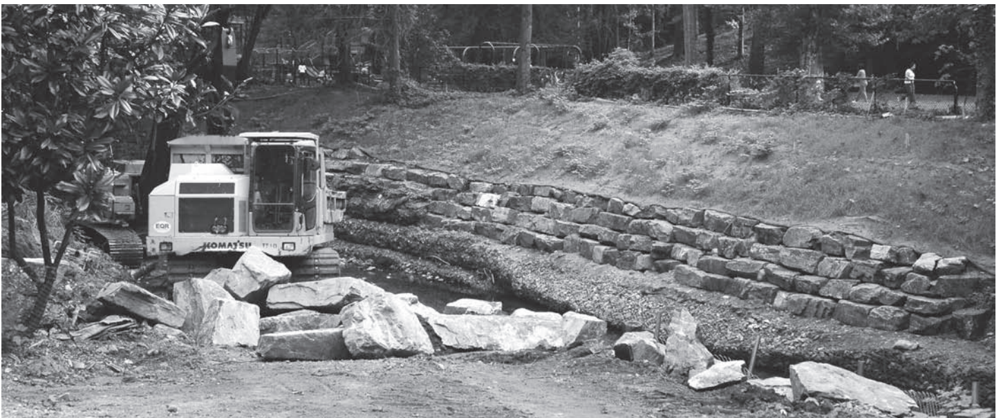
Construction machines put rocks in place as part of Stony Run restoration near Linkwood Park.
